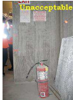
Improper floor placement of Fire Extinguisher.
